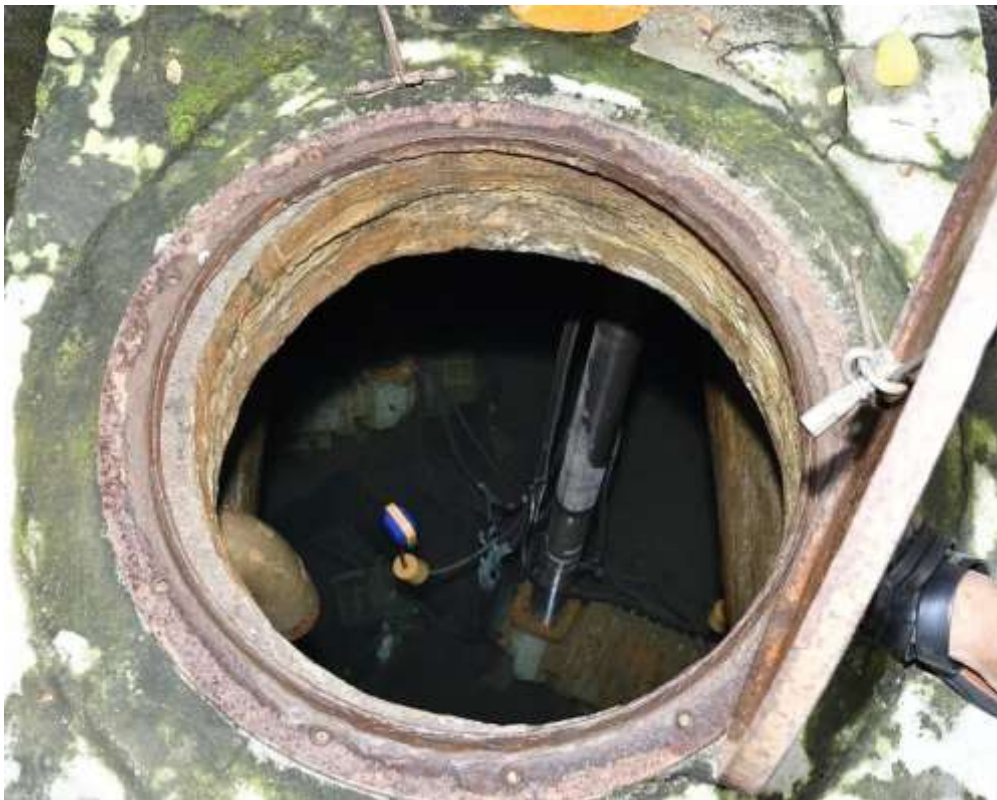
Underground Water Tank
